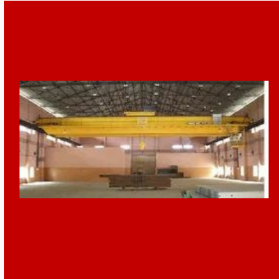
Double Girder EOT Cranes
